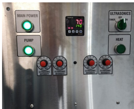
Figure 21 Pump Manual Control On
