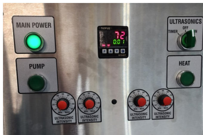
Figure 9 Ultrasonic Generators Turned Off
