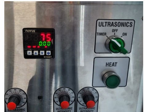
Figure 14 Generator Timer Cycle Done
