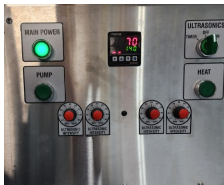
Figure 20 Pump Manual Control Off
